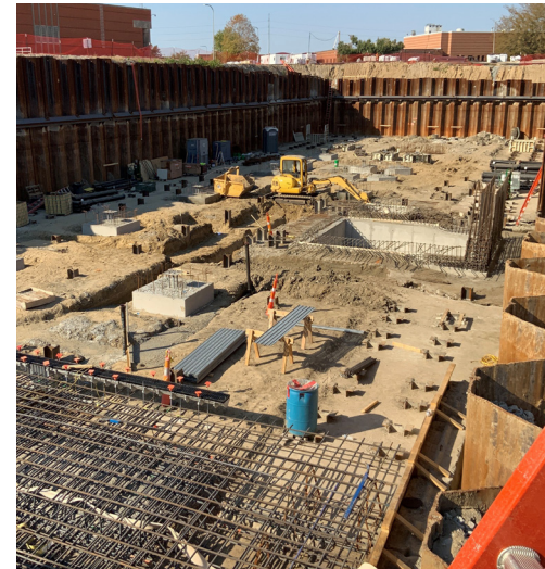
Bissell Wastewater Treatment Plant, October 2024: Solids Processing Building excavation and foundation construction. Completed elevator pit visible in center of basement.
