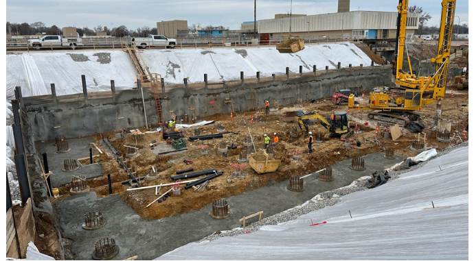
Lemay - Drilled Shaft construction in progress, an below slab drain piping installation.
