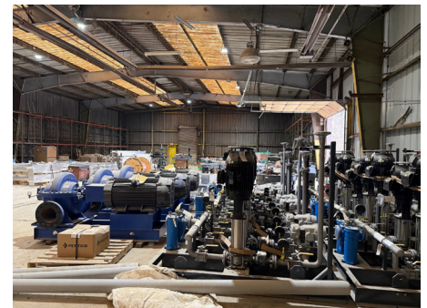
Process equipment, including pumps and assemblies, is received and staged in storage for future installation.
