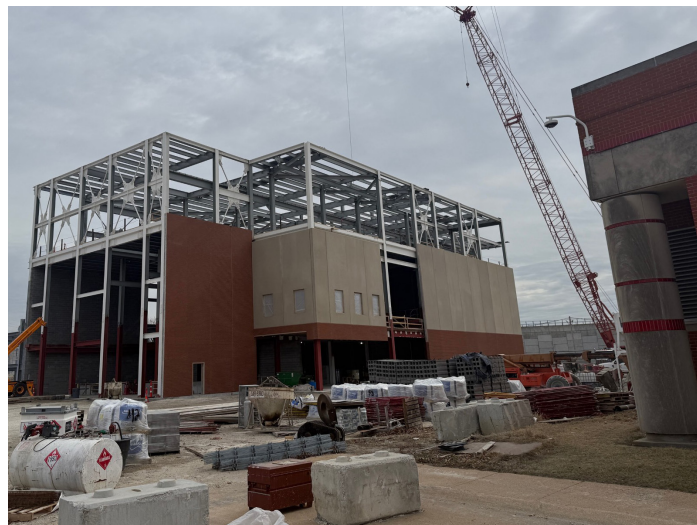
Structural steel erection and exterior wall panel installation progress on the Bissell SPB.
