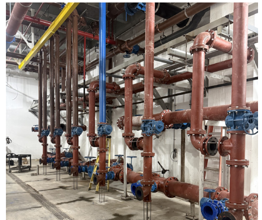
Bissell — process piping for raw sludge.
